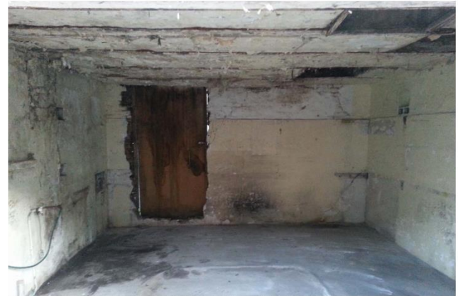
Figure 11: - Site Photograph - existing building in a state of disrepair
