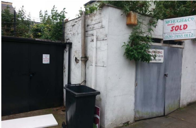
Figure 10: - Site Photograph - Dead zone - could be used for anti-social activities
